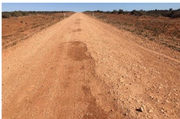
Figure 6: Anabranch Mail Road - poor pavement condition
