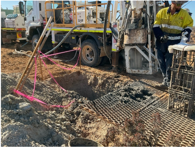
Figure 4 Water injection on the cyclone above the small sump collecting drill cuttings
